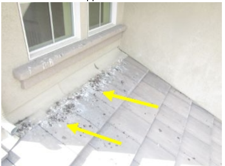
Bird droppings noted
