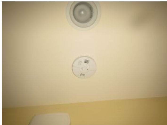
Combination smoke detector and carbon monoxide sensor noted
