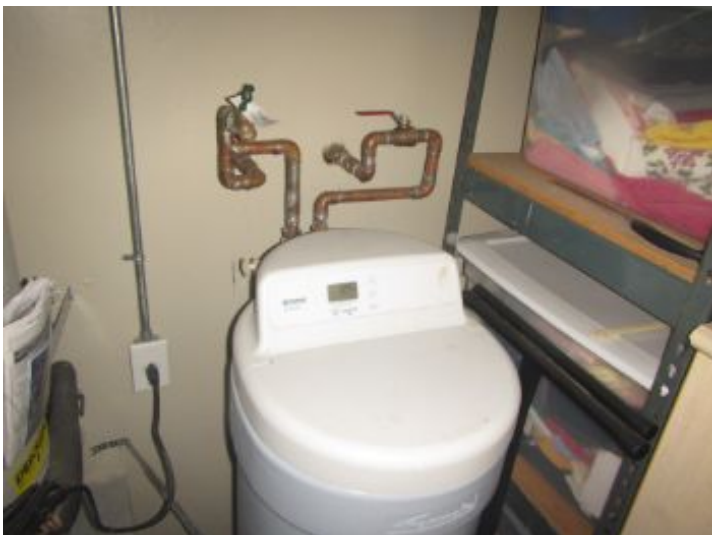
Water softener noted
