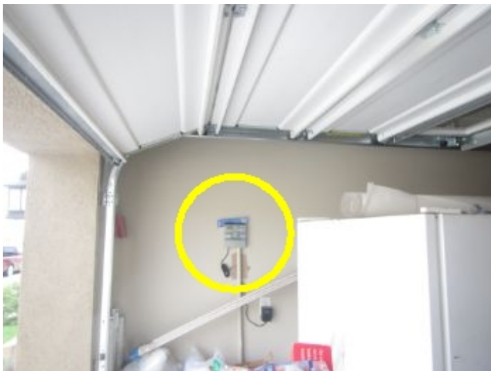
Sprinkler timer noted
