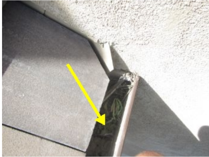
Recommend cleaning out the gutters
