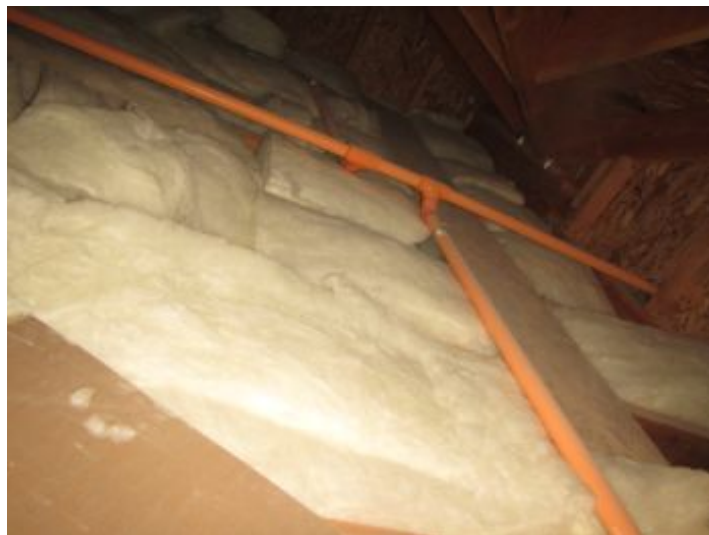
Fire sprinkler plumbing noted
