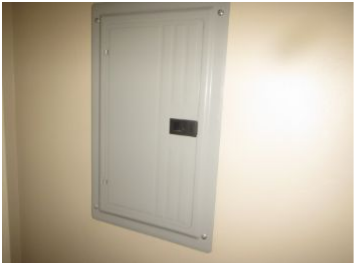
Subpanel located in the laundry room
