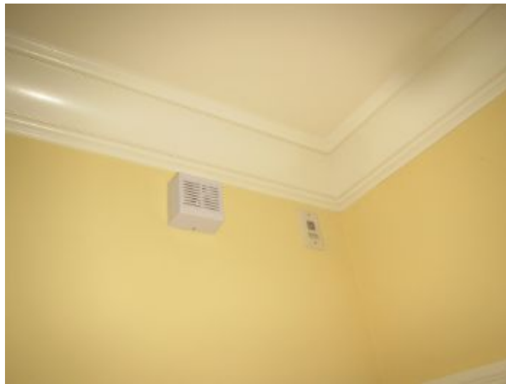
Fire detector noted
