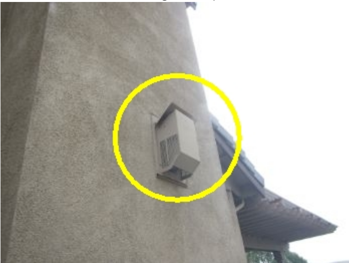
Vent for gas fireplace noted
