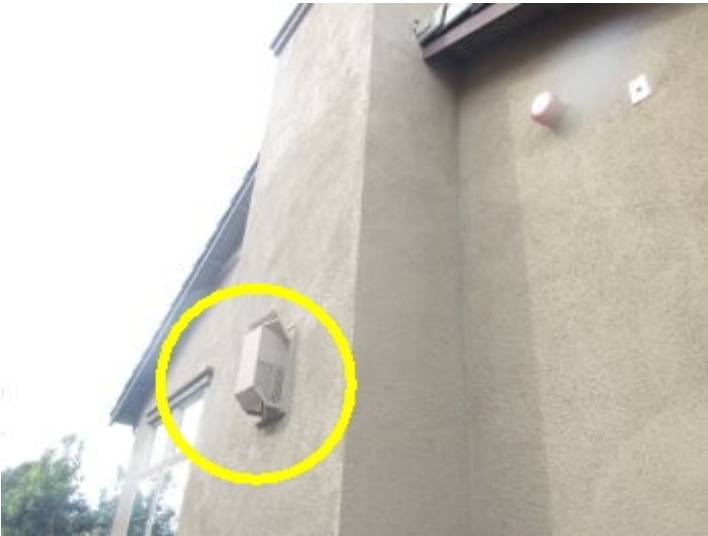
Direct vent for gas fireplace noted
