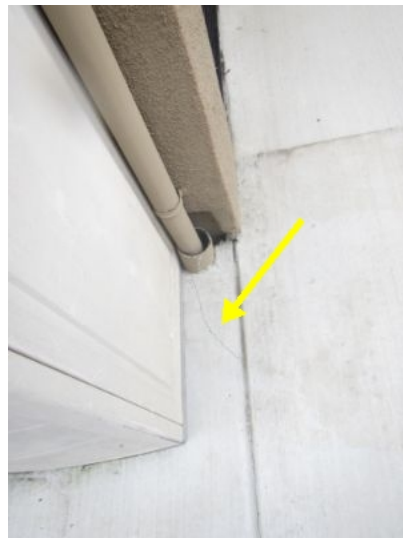
Common crack noted
