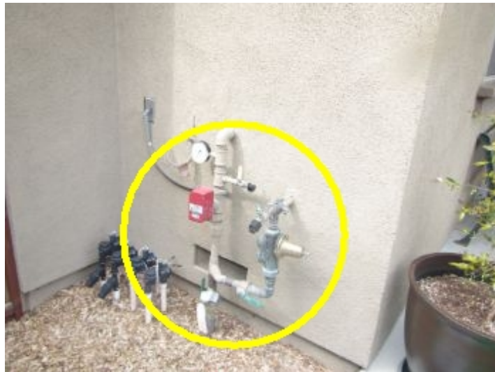
Pressure regulator, main water shutoff and fire sprinkler main valve noted
