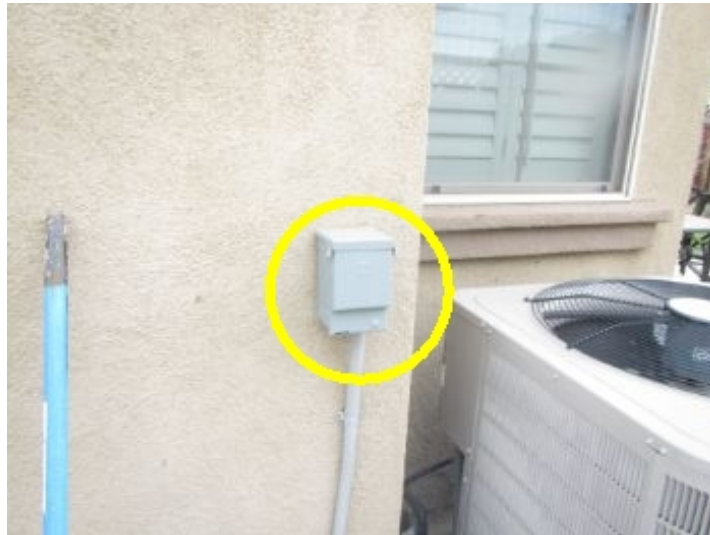
Service disconnect for A/C unit noted
